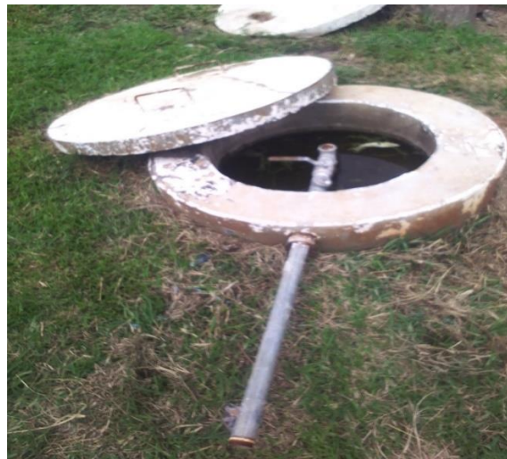
Fig. 5. Example of a fixed dome biogas plant as captured at Manchinci Sewage Treatment Plant under Lusaka Water and Sanitation Company Limited
